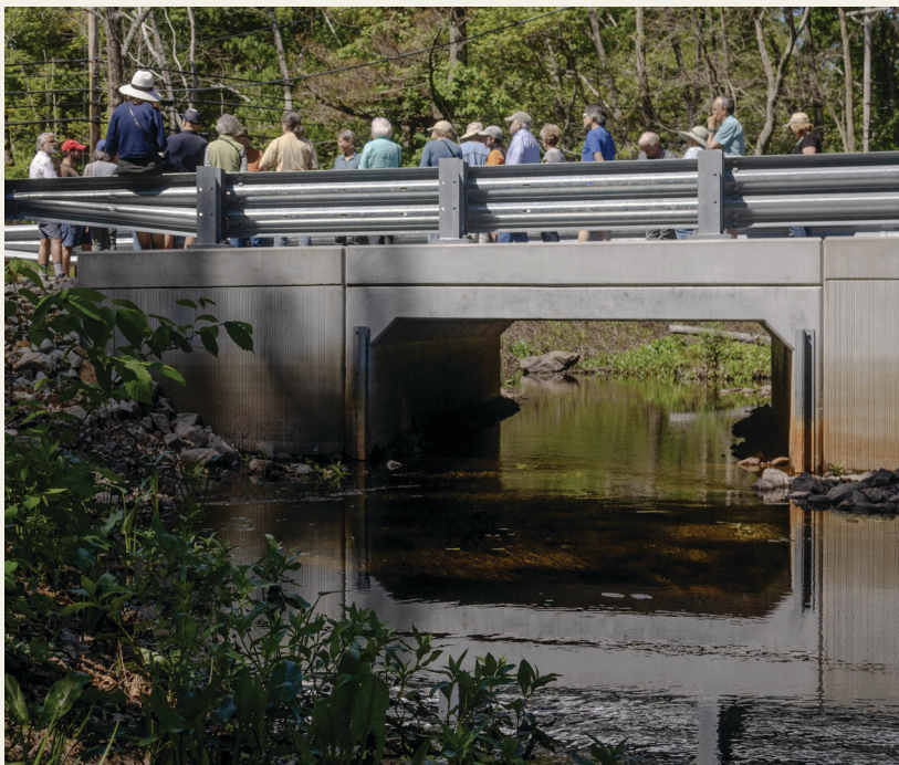
Recently built culvert that serves flood and habitat protection needs. Photo by Amanda Siow, 2024
