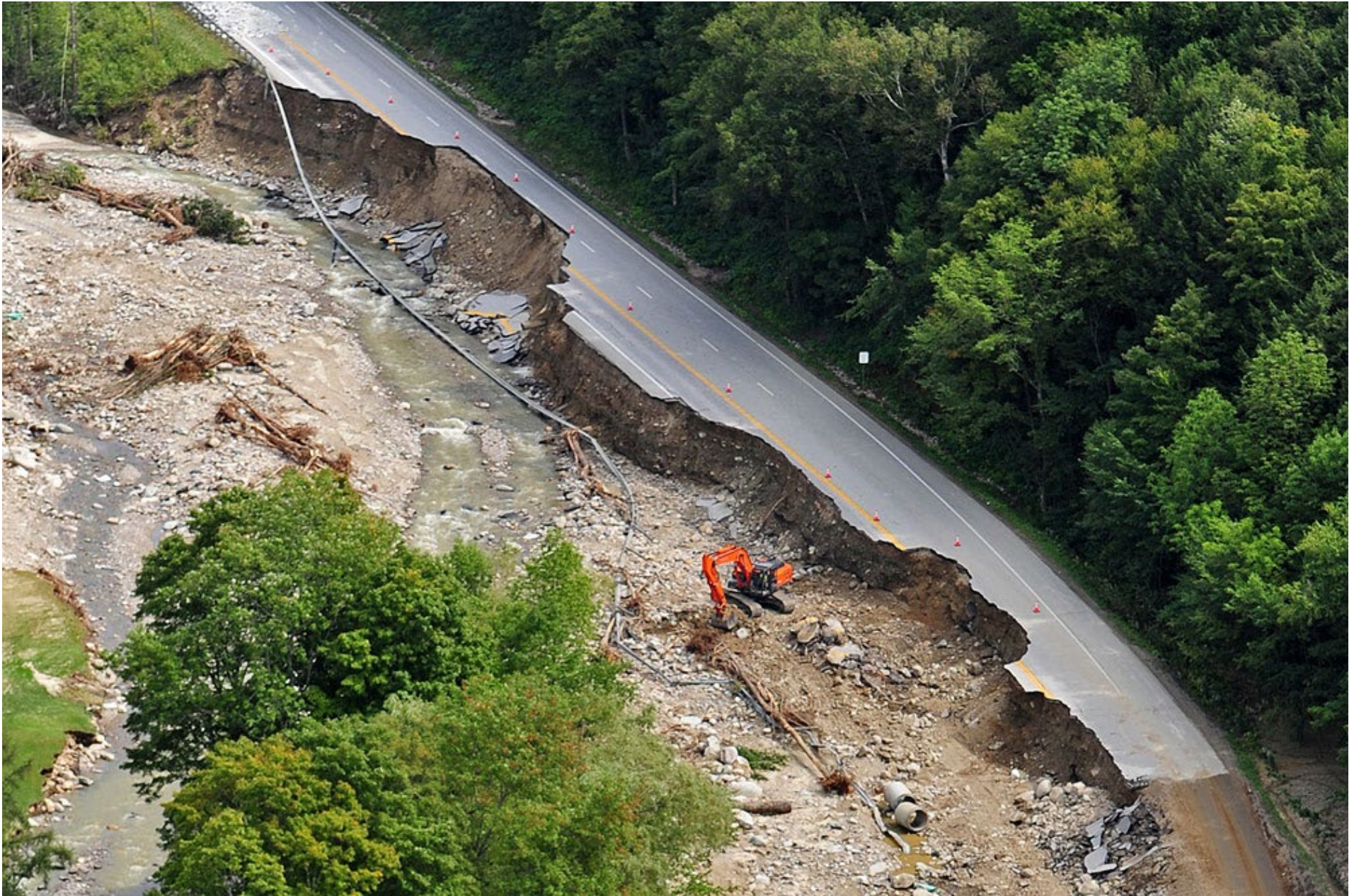
Hurricane Irene damage on Vermont Route 107 (VTRANS, 2011)
