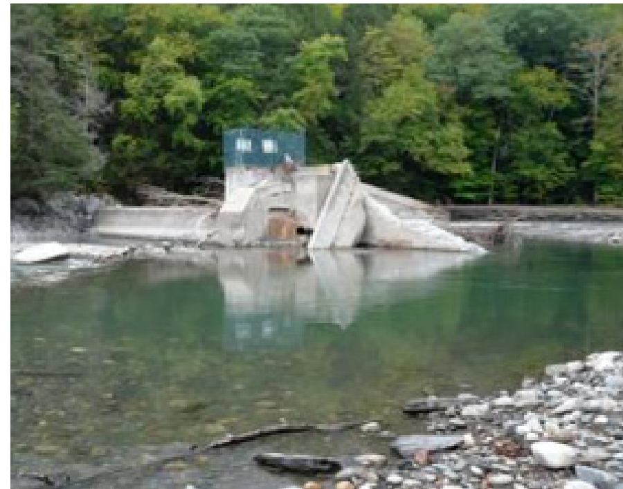
Failed dam on the Green River in Massachusetts shows the river flowing around the spillway and through the retaining wall breach.
