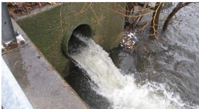
Combined sewer overflow in Mystic River watershed (Courtesy of MyRWA)
